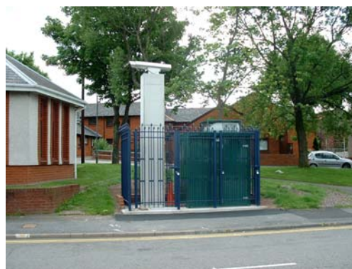
Photo 2 - St Thomas DOAS Receiver Station
